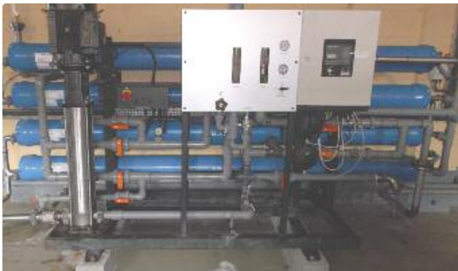
Reverse osmosis equipment at Camerons Brewery, Hartlepool.
