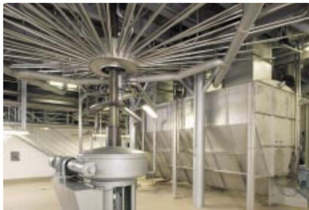
Figure 7: The underside of a modern lauter tun – take note of the number of wort run off pipes – photo supplied by Huppmann
